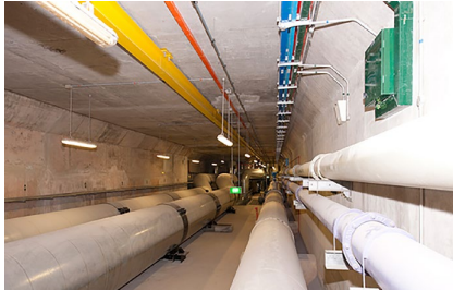
Abb. 04: Common Service Tunnel (CST) [Foto: © ctrlshift.gov.sg 16 ]
