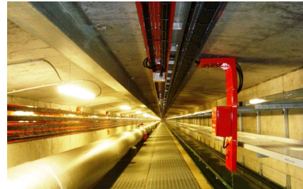
Abb. 05: Azabu-Hibiya Common Utility Tunnel [Foto: © tokyoreporter.com 17 ]
