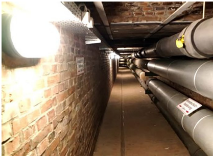
Fig. 02: Utility Tunnel in Dresdner Old Town [Source: © GIBA mbH]
