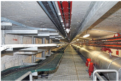
Fig. 06: Common Utility Tunnel (CUT) [Source: © The Star.com.my 19 ]
