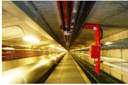
Fig. 05: Azabu-Hibiya Common Utility Tunnel [Source: © tokyoreporter.com 18 ]
